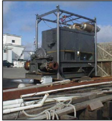
Figure 11. Pump with diesel engine
